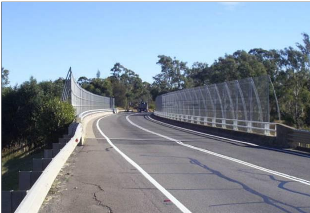
Figure 5.2 – Limited Pedestrian Clearance on Menangle Road Bridge
